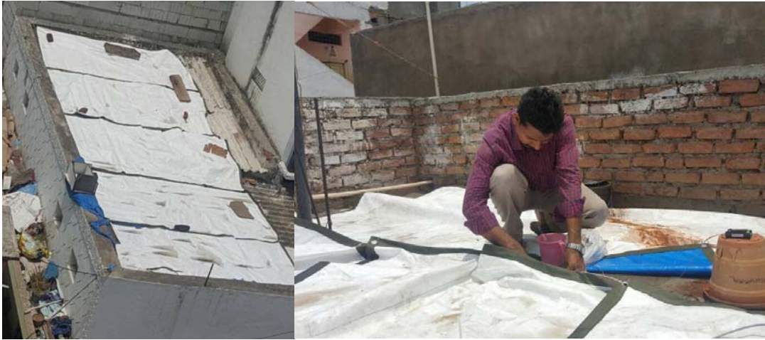
Figure 7: Pictures showing cool roof pilot installation and testing underway in Hyderabad, May 2017 (NRDC)
